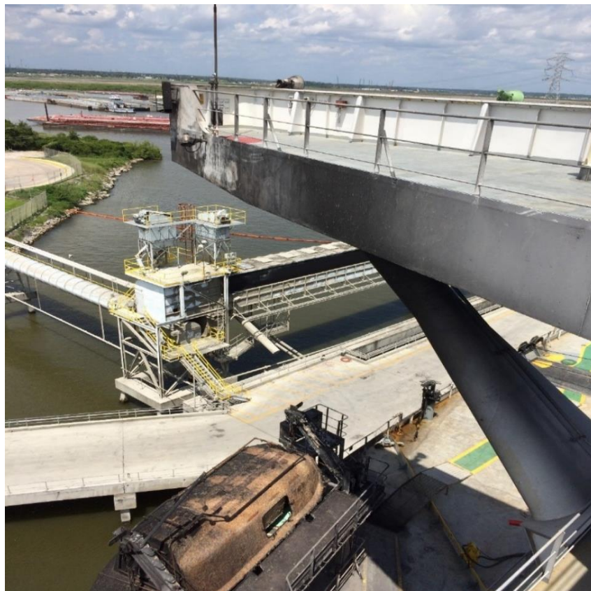
Fire damage to Aframax River 's portside bridge wing (where the conning pilot was standing when the fire erupted), lifeboat, and main deck.
