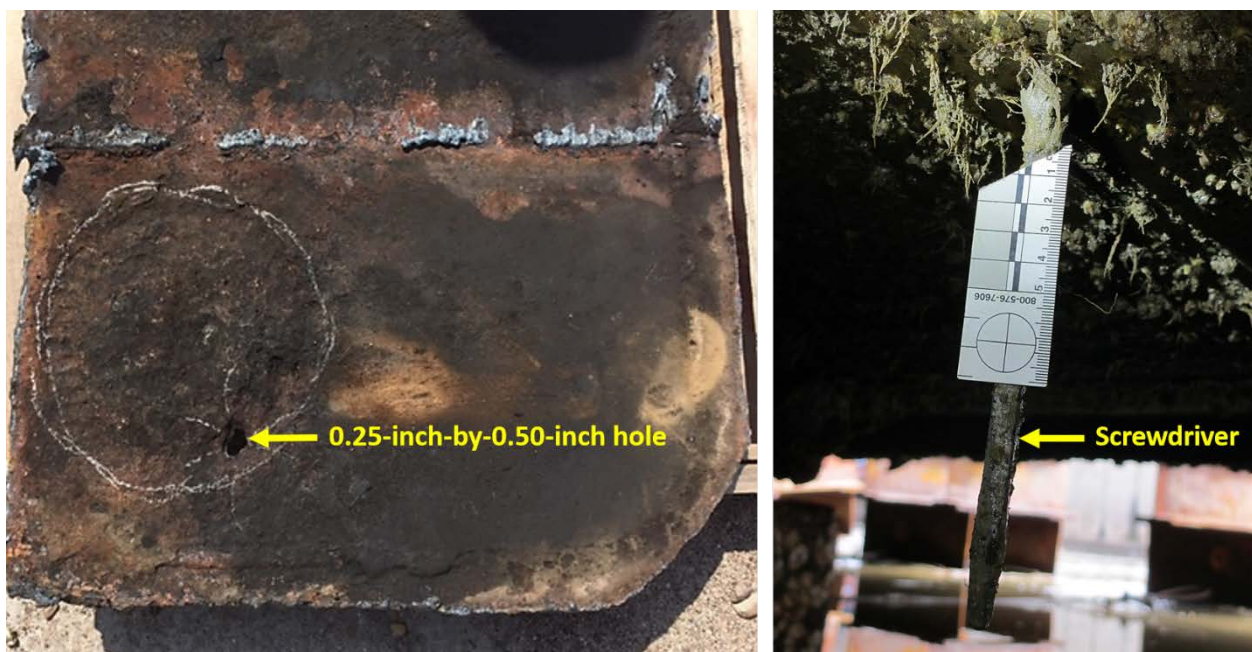
At left, the hole found near frame 31 of the bottom plating. At right, the screwdriver placed in the hole as a temporary repair. (Photos by Coast Guard)
