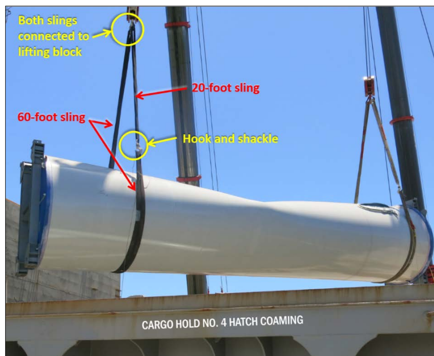
Removal of the damaged tower base section by a shore-based crane mirrors the lifting arrangement used by the vessel's cranes at the time of the accident.
