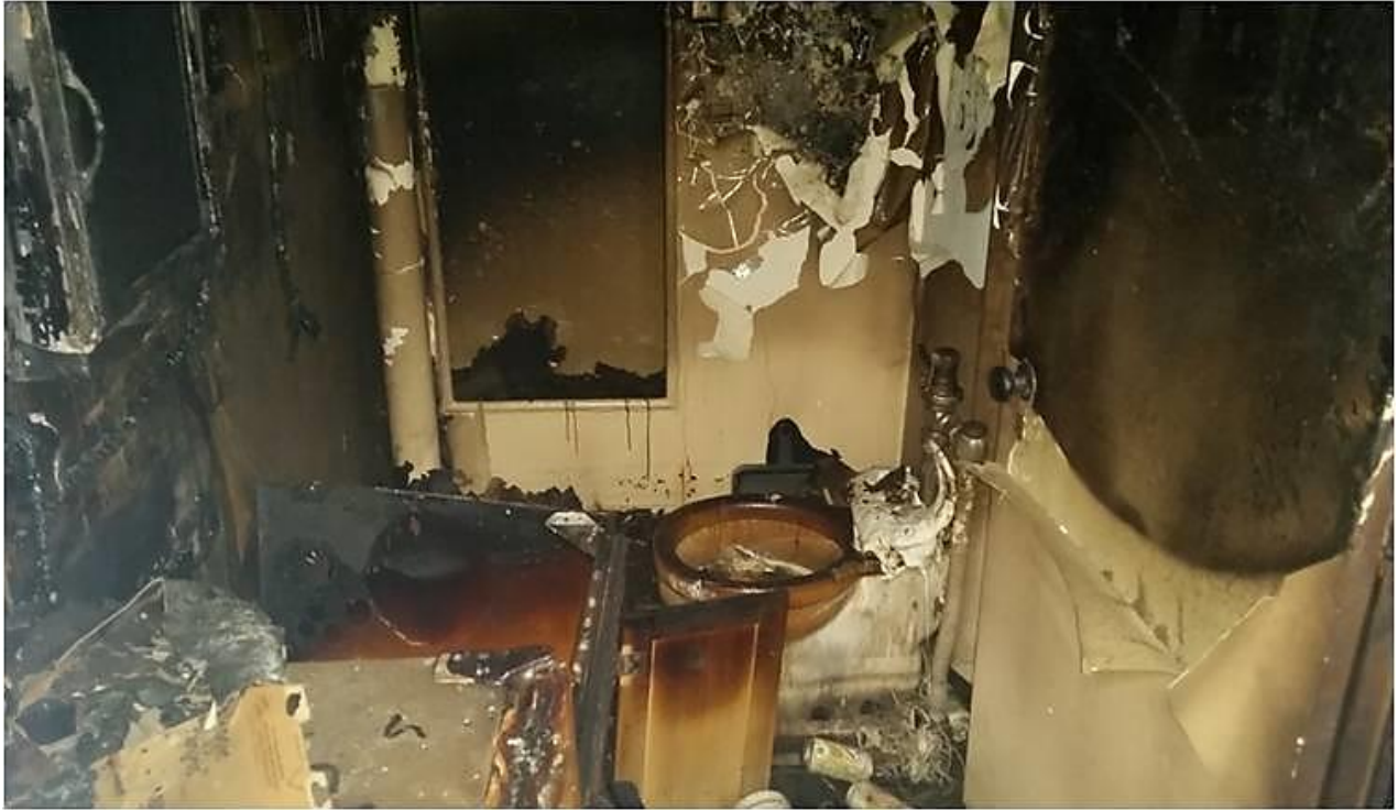
Fire damage to one of the Alpena bathrooms. (Photo by Coast Guard)
