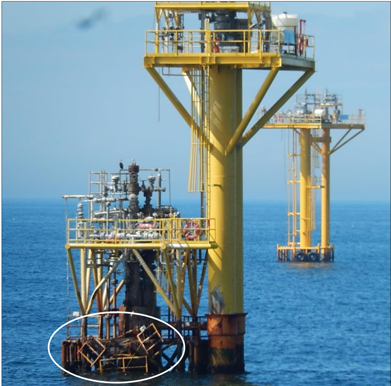
Displaced rails, catwalk, and risers on natural gas production platform Ship Shoal 119 W. (Photo provided by the Coast Guard)
