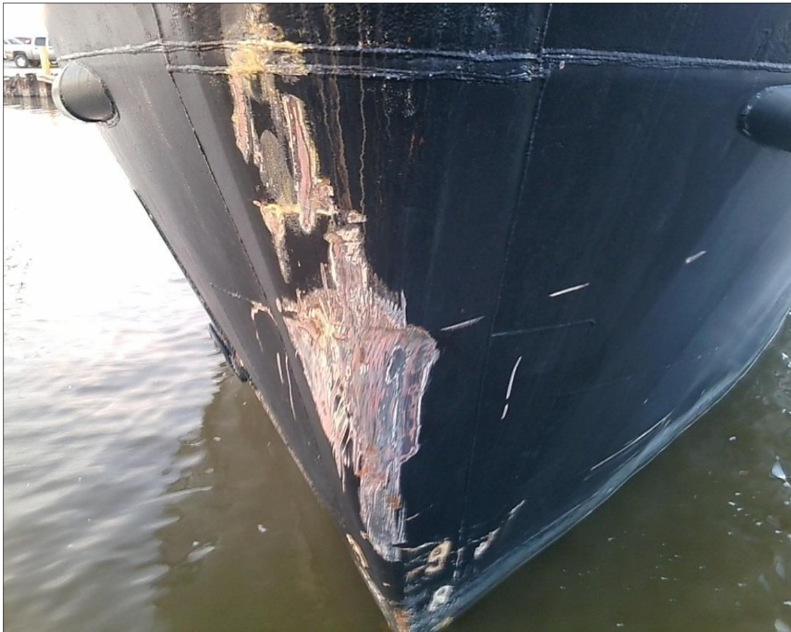
Damaged bow of the Tristan Janice . (Photo provided by the Coast Guard)
