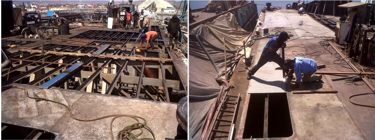
Barge Nash in the Ensenada shipyard during renewal of main deck plating. (Photos by SBBL)
