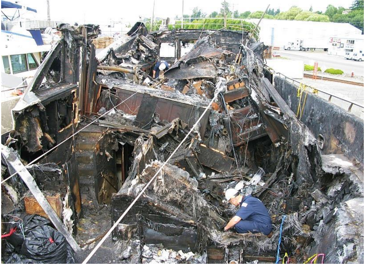
Looking aft from the vessel's forward end at the burned and melted fiberglass hull and interior.
