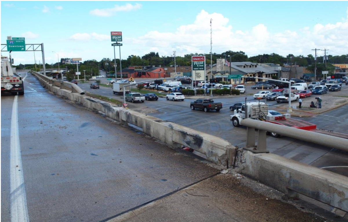
Figure 3. Bridge rail after being struck by the HISD school bus (view is to the southeast).
