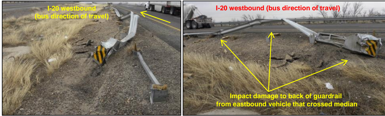
Figure 3. Condition of guardrail along I-20 westbound on January 13, 2015, after it was struck by eastbound vehicle and moved off roadway. (Source: TxDOT)
