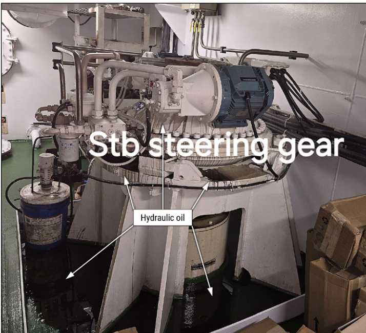
Jack Edwards starboard steering gear as found immediately after collision.
