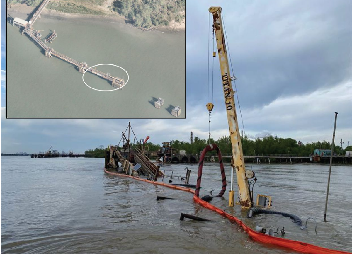
The collapsed crude oil dock, looking upriver. Inset shows the area of the dock that collapsed (circled). SOURCES: COAST GUARD, NEARMAP.
