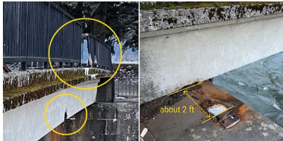
Damage to the pedestrian bridge deck and railing (circled) and displacement of the deck. BACKGROUND SOURCE: PORT OF CASCADE LOCKS PORT COMMISSION.
