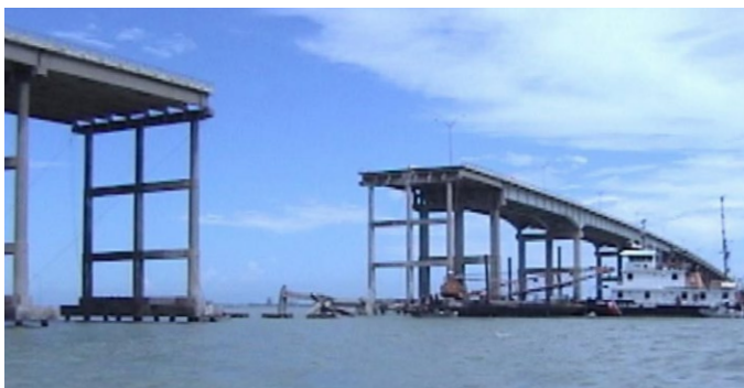
Collapsed section of Queen Isabella Causeway in Port Isabel, Texas. On September 15, 2001, four loaded barges crashed into one of the bridge's support columns. The collision caused two 80-foot spans to fall into the water. Eight people were killed as their cars fell 85 feet into the water. Five vehicles were recovered from the water along with three survivors.
