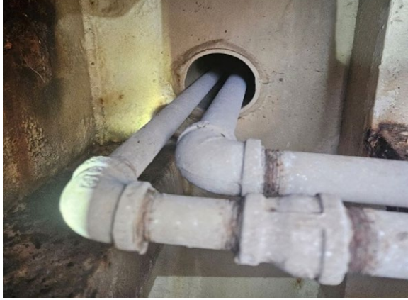
View of unsealed piping conduit penetration between the engine room and auxiliary space from the auxiliary space on May 28, 2024. SOURCE: COAST GUARD.
