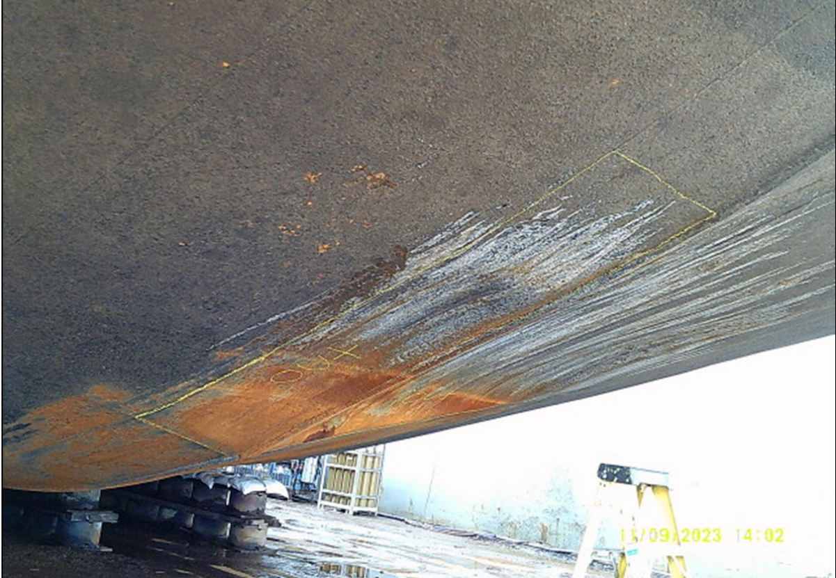
Bottom plating near the bow of the John M Donnelly that was inset when the vessel grounded.
