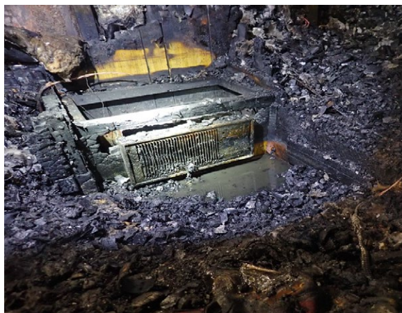
Electric heater in first mate's stateroom after the fire.
