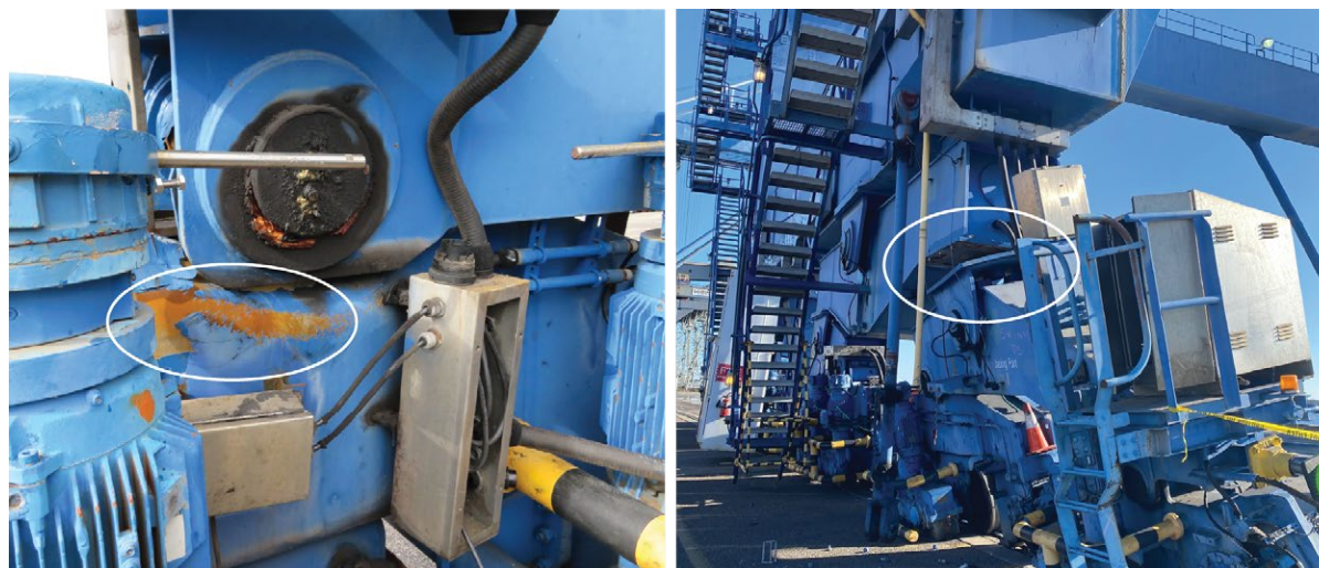
Left to right: The damaged STS crane. Circled areas show (1) metal distress and (2) damage to one of four gantry assemblies.
