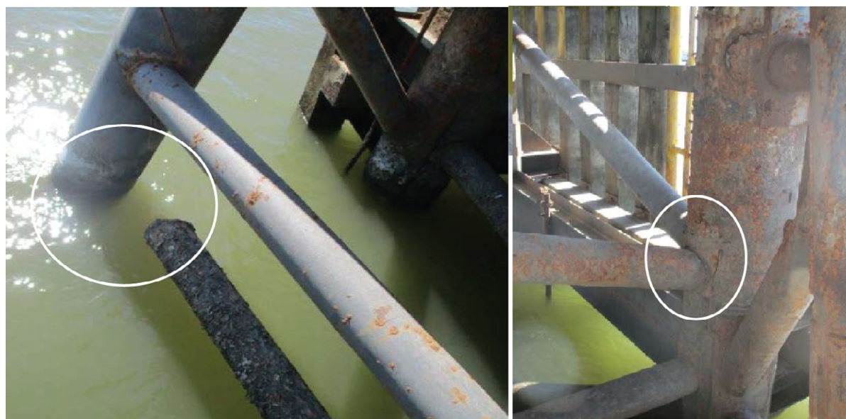
Visual inspection photos from 2021 showing a lower header joint not connected to the other column and a joint starting to disconnect on the dolphin no. 3 transfer platform at the Chalmette Refinery crude oil dock.
