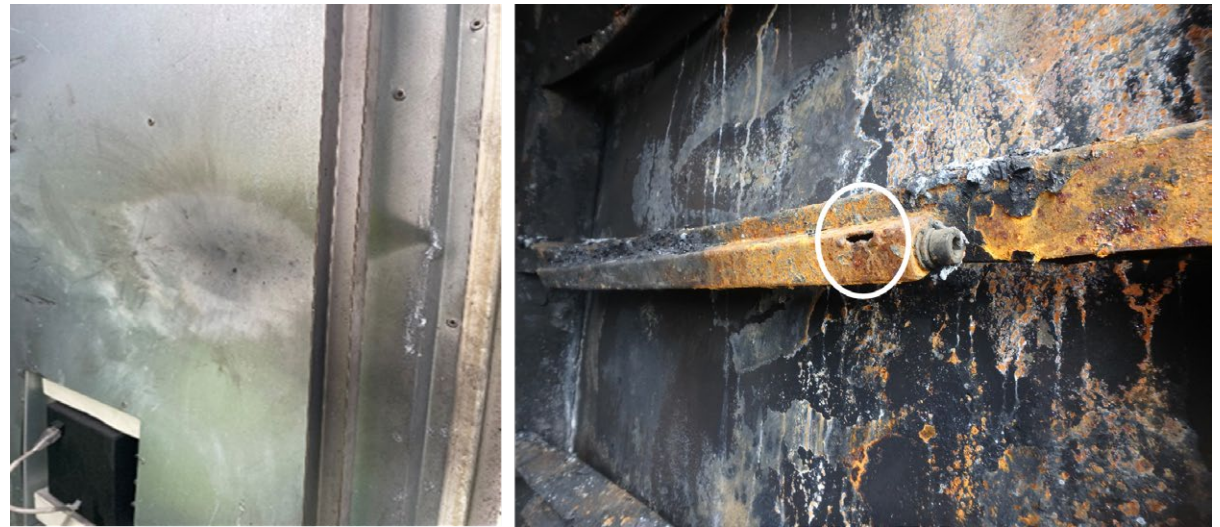
Examples of internal damage due to indentation and scorching, and arcing (circled) found inside of the BESS units on the tween deck in cargo holds no. 1 and no. 2. BACKGROUND SOURCE: ESA.
