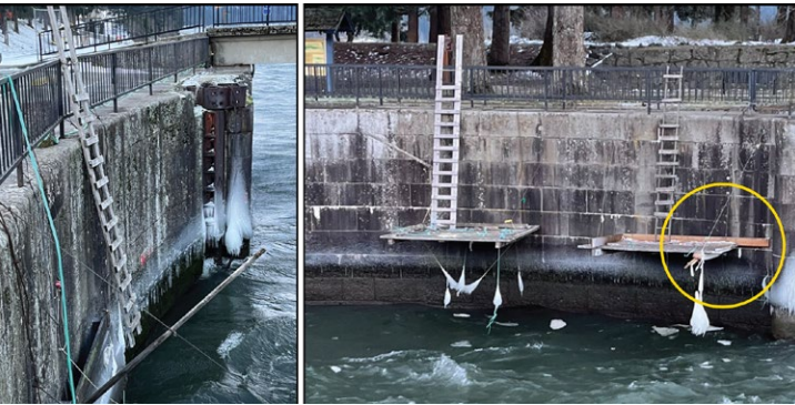
The area where the destroyed fishing platform had been mounted and damage to one of the platforms on the opposite side of the lock (circled).
