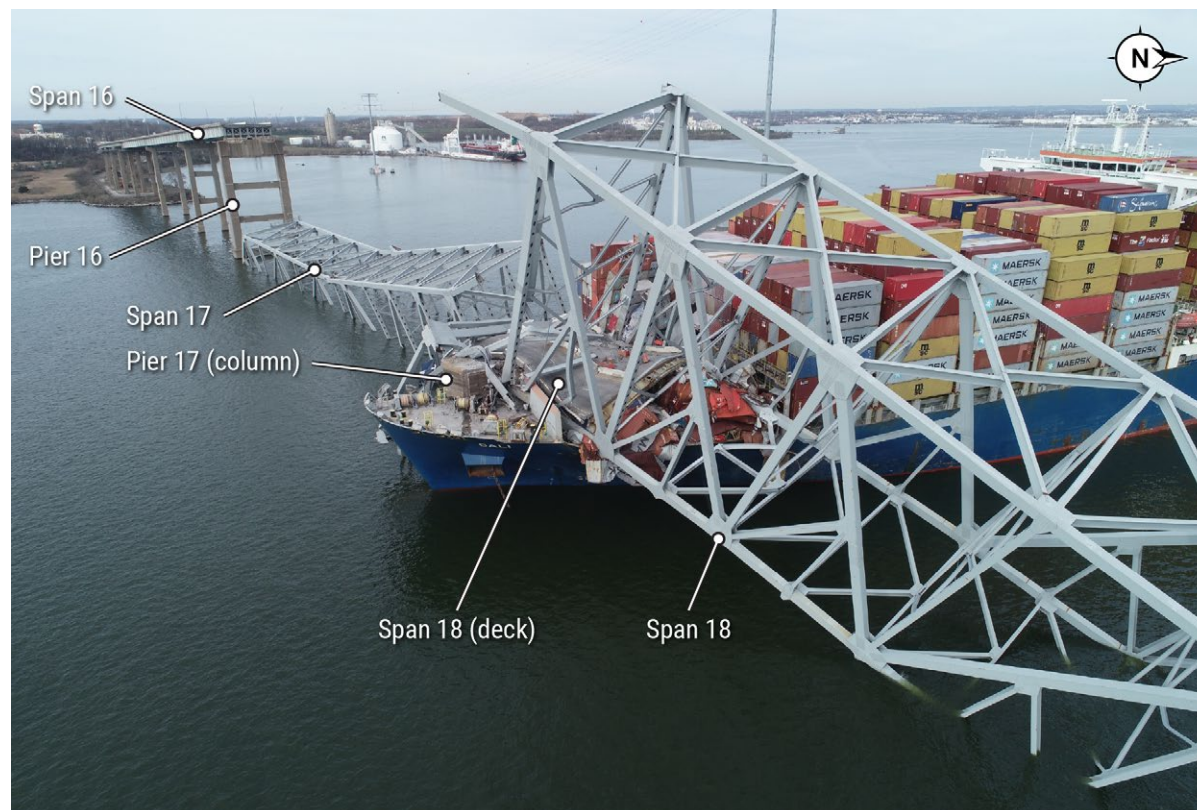
Damage to bridge Spans 16–18 and Pier 17, as seen looking toward the port side of the Dali .
