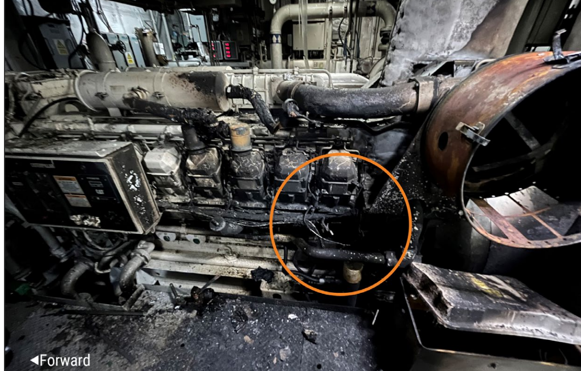
Damaged no. 2 auxiliary generator aboard Ocean Navigator after the engine failure. The circled area identifies the location of the engine block damage.
