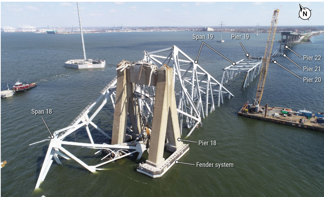
Damage to Spans 18 and 19, and Piers 18–22.
