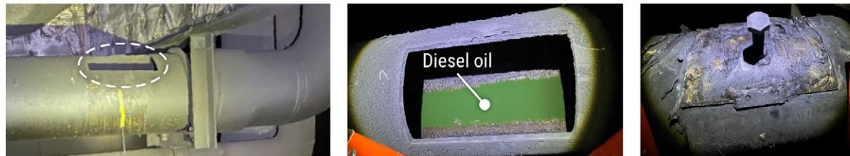
Left to right: Circled area identifying the open section of fuel vent piping on D deck; diesel oil observed in vent piping, seen from above, through cut out section; and cut out placed back in position.
