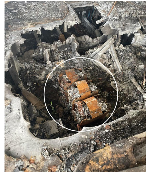
The 24-volt lithium-ion battery bank (circled), after the fire.
