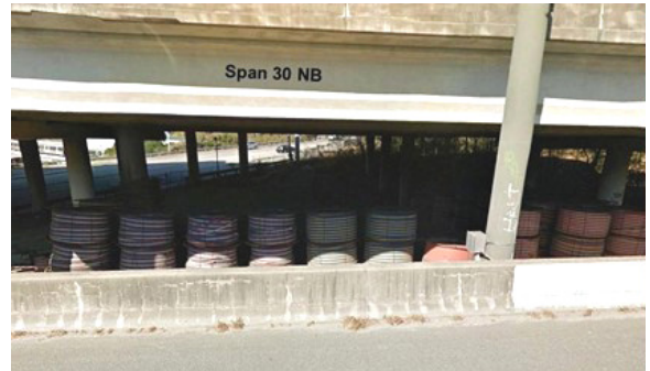
Prefire storage area under span 30 NB of the I-85 bridge, showing numerous reels of high-density polyethylene conduit.
