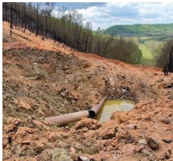
Figure 31. Ruptured Enbridge Inc. pipeline in Hillsboro, Kentucky, following the release and ignition of natural gas. SOURCE: BGC ENGINEERING USA INC.
