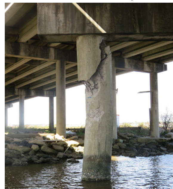
Figure 105. Below: Damaged section of struck pier column under westbound lanes of I-10 bridge.
