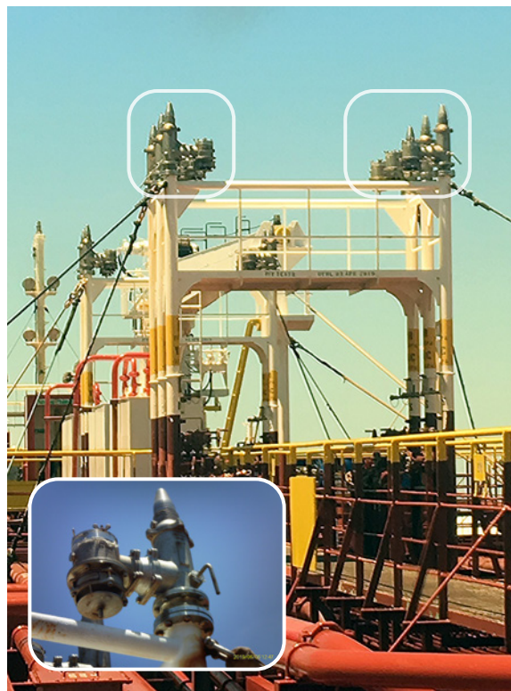
Figure 183. PV valves on board the main deck of the Fairchem Filly .
