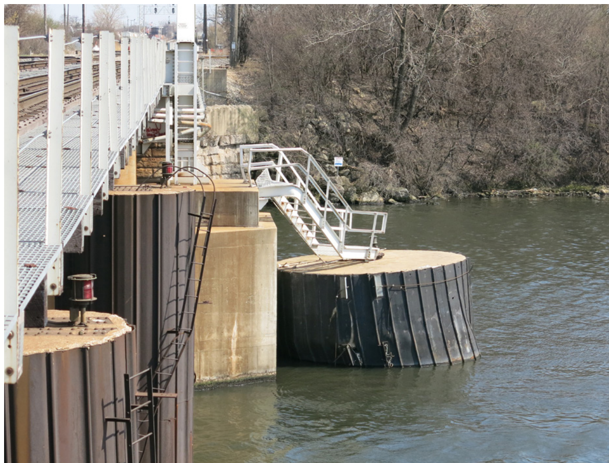
Figure 71. Below: Postaccident condition of the south side of the CSX Railroad Bridge.
