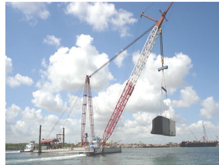
Figure 156. Atlantic Giant II prior to accident.
