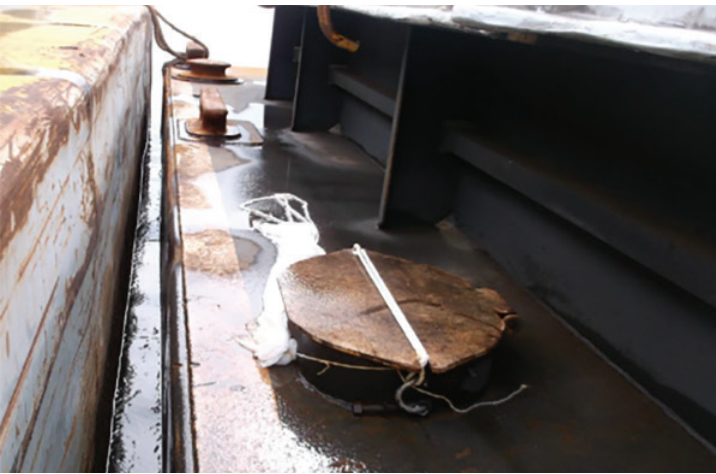
Figure 135. Postaccident views of a manhole cover on the PTC 625 is in poor condition, with missing dogs, and strapped down with line.
