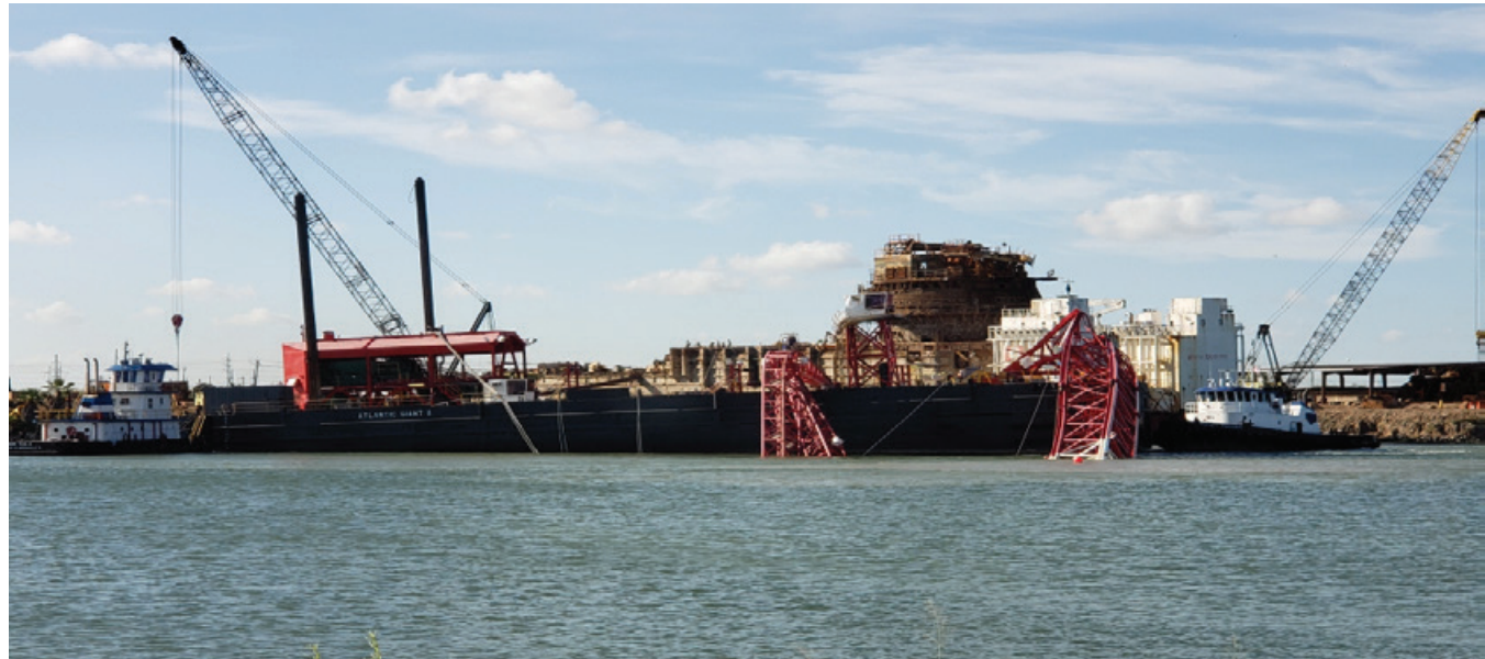
Figure 153. Collapsed crane boom on Atlantic Giant II . In background are TOPS DB1 and BOABARGE 29 .
