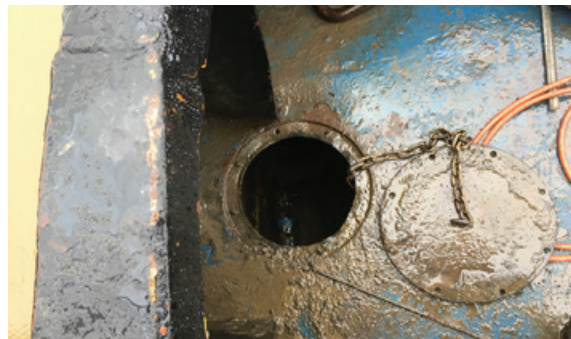
Figure 130. Starboard deck access to aft stern void found open during salvage, with broken and missing access cover screws.
