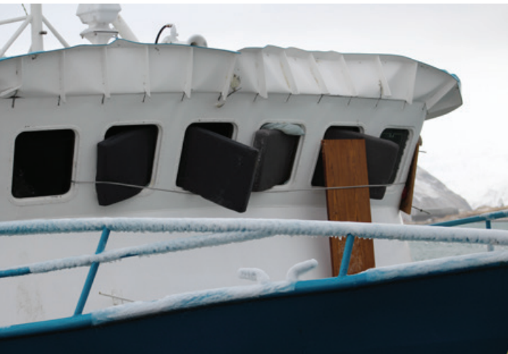
Figure 157. Wheelhouse damage and missing windows on the Progress .
