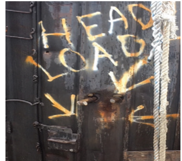
Figure 51. Below, the forward piling at Jacks Run with a broken mooring ring anchor point and missing ring.
