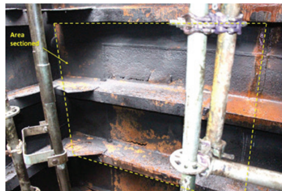
Figure 75. Cracks in bulkhead separating the forepeak from the port no. 1 cargo tank. The dashed section was removed and sent to the NTSB Materials Laboratory for analysis. SOURCE: COAST GUARD
