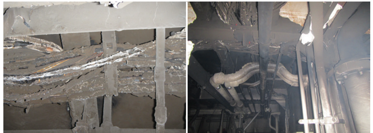
Figure 80. Left: Electrical cabling above generator no. 2. Right: Smoke and heat damage in the overhead of the starboard forward corner of the lower engine room. SOURCE: COAST GUARD
