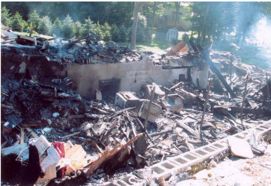
Figure 1. Damage to 48 Woodland Lane.
