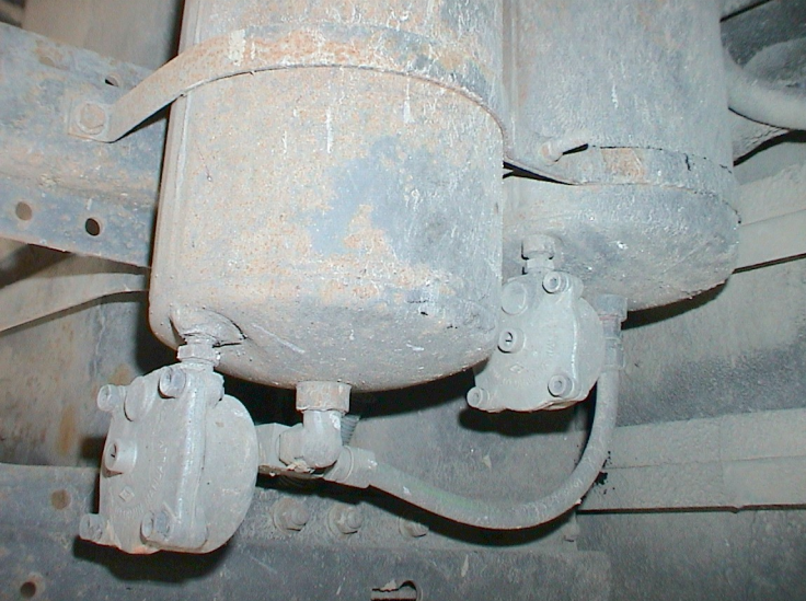
VEH Photo #14 - Right Front Air Tanks Showing DV-2 Automatic Drain Valves
